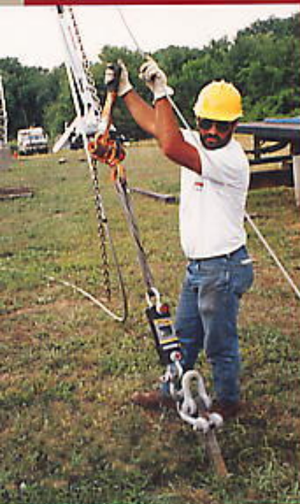
▲ Dyna-Link in use to monitor tower line tension.
